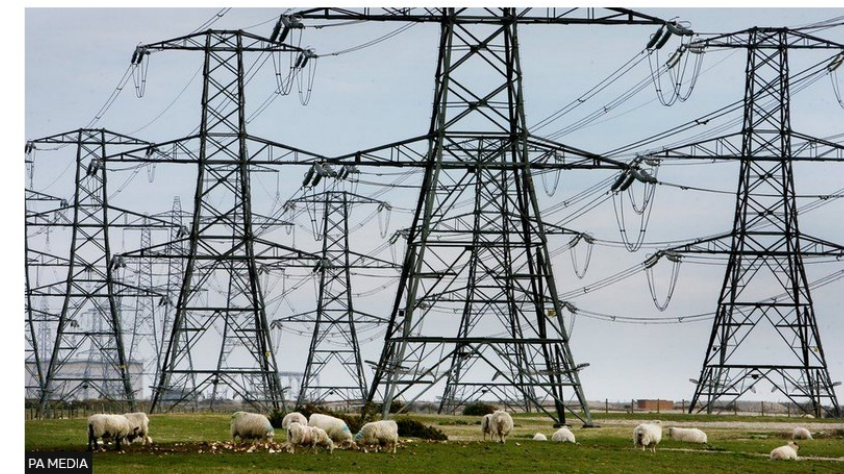
PA MEDIA Northern Powergrid is responsible for providing power to 3.9m households in the North East, Yorkshire and northern Lincolnshire
