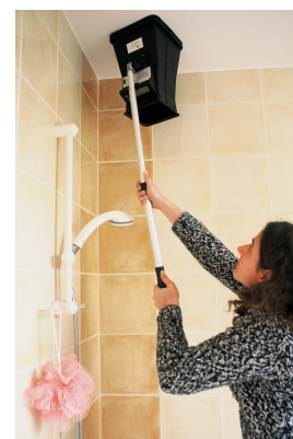
Measurement of the extracted air flow at extraction openings
