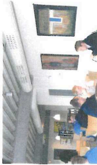
FIGURE 30. Duct diffuser installed in a restaurant.
