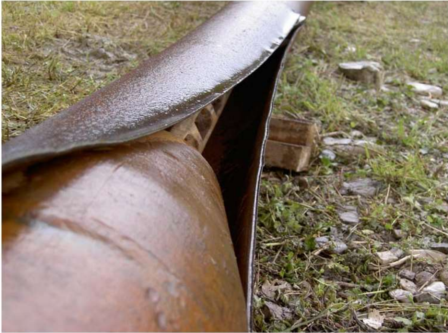
close-up of pipe splitting
