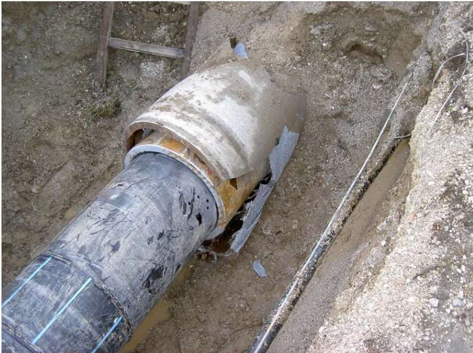
initial phase in replacement of an asbestos cement pipe using the pipe bursting technique
