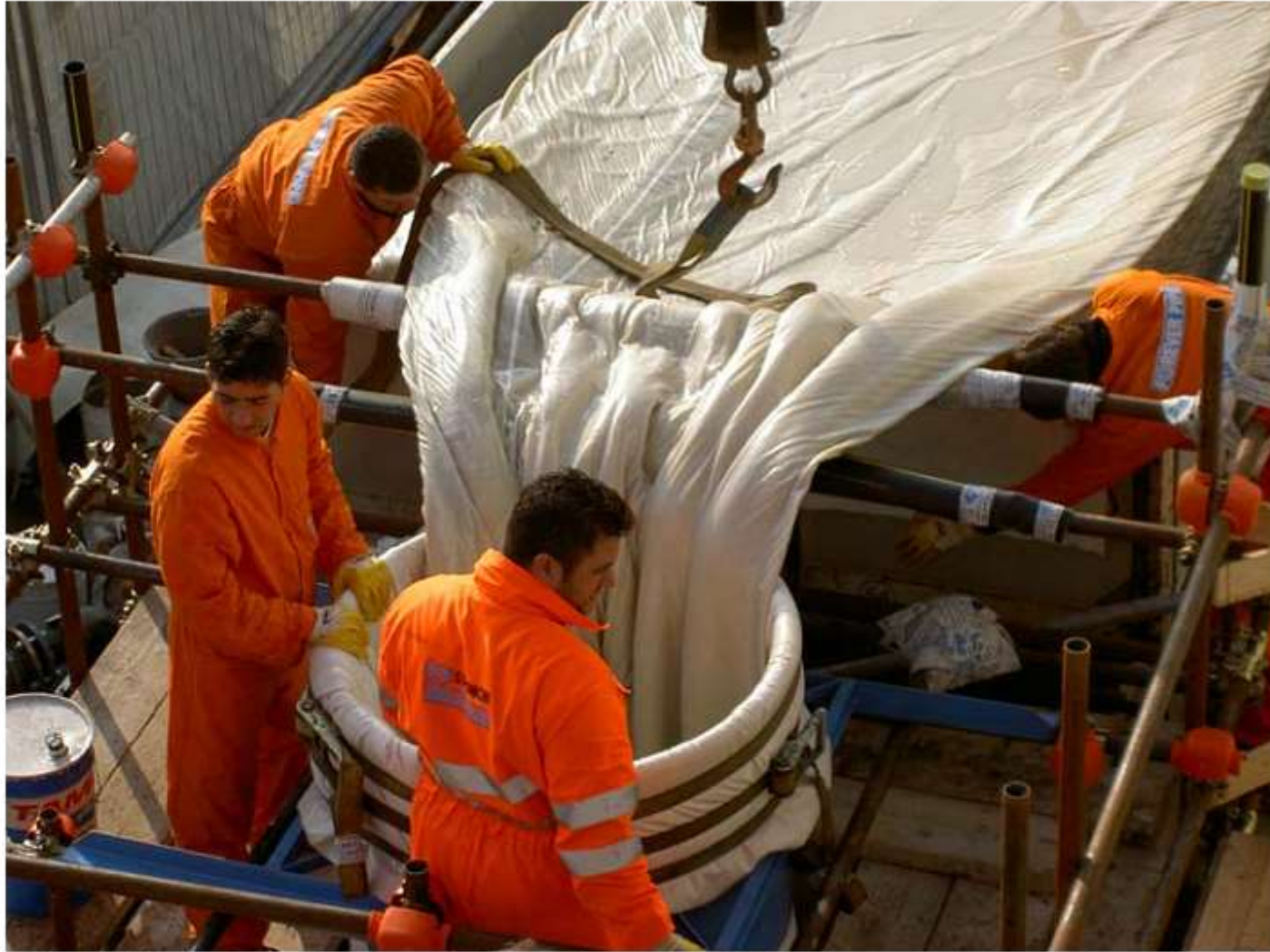
insertion of the tube impregnated with resin and cooled, after anchoring the inversion flange
