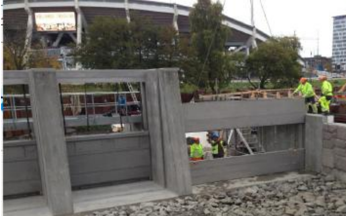
2404 used in water gates to regulate the river through Gotemburg.
