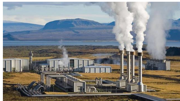
Figure 5: The Olkaria Geothermal Power plants
