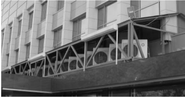
Figure 6.1 Air conditioners installed on the Central Universal Department Store (TSUM) in Tomsk, Siberia. While winter temperatures can drop below -40^{\circ}\text{C} , summers can be quite balmy. Photo by David Banks.
