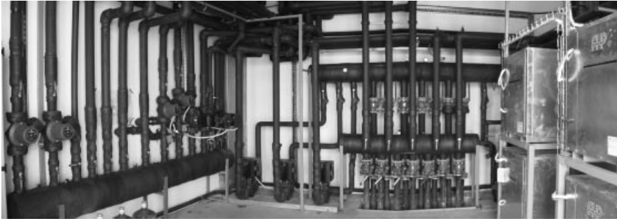
Figure 9.1 A ground source heating and cooling plant room at a car showroom in Bucharest, Romania, showing manifolds, fluid circulation pumps (left) and an array of heat pumps (right). Reproduced by kind permission of ASA Georexchange SRL, Bucharest.
