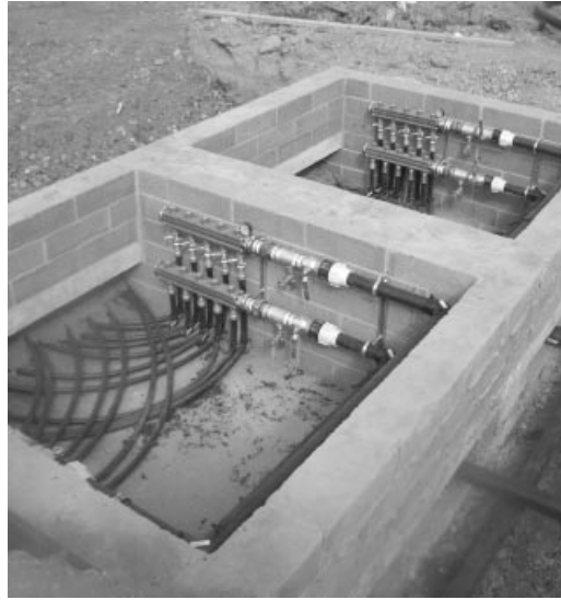
Figure 9.10 A rather complex arrangement of carrier fluid manifolds in a subsurface chamber; photograph reproduced by kind permission of Geowarmth Heat Pumps Ltd.
