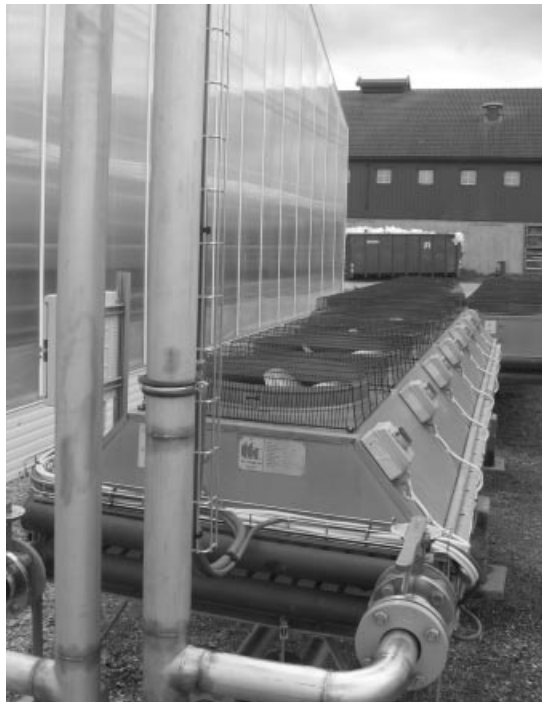
Figure 6.3 An array of dry coolers in Norway. A hot fluid (which is to be cooled) circulates through a radiator grid below the horizontal fan elements. Photo by David Banks.
