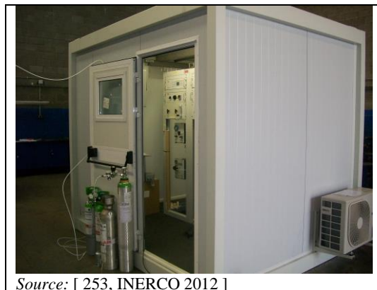
Figure 4.3: Example of air-conditioned housing for an AMS
