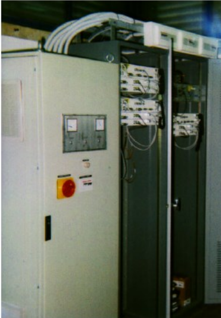
General power supply and radio apparatus for communication towards Cesena and Forlì
